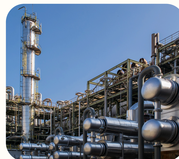
Produced Water Treatment
